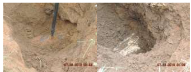
Figure 3.1 Sight of probed disuse 5.5”Apara gas pipe (left) and life 6” gas pipe (right)
